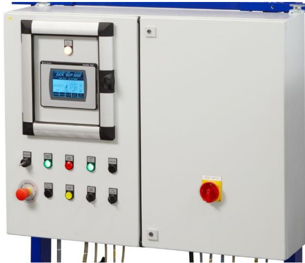
Fig. 13: Control and power supply cabinet
