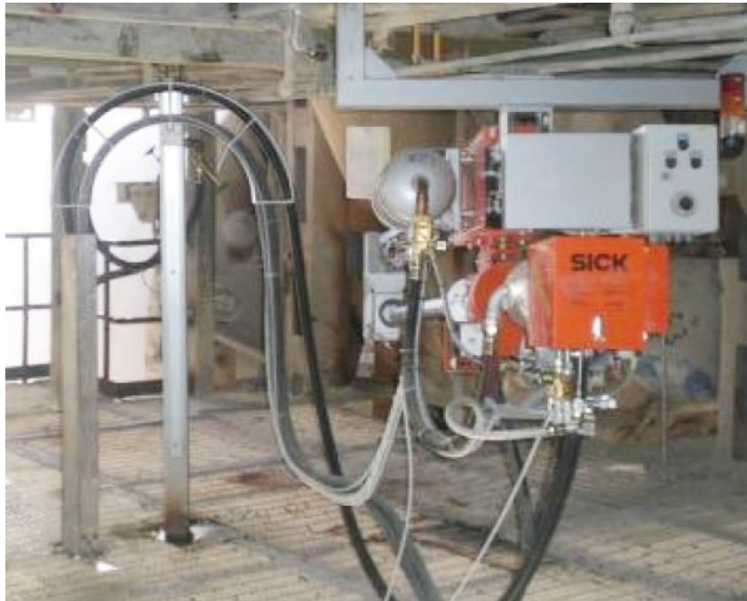
Fig. 31: Hose support on a mast and on the floor (example)
