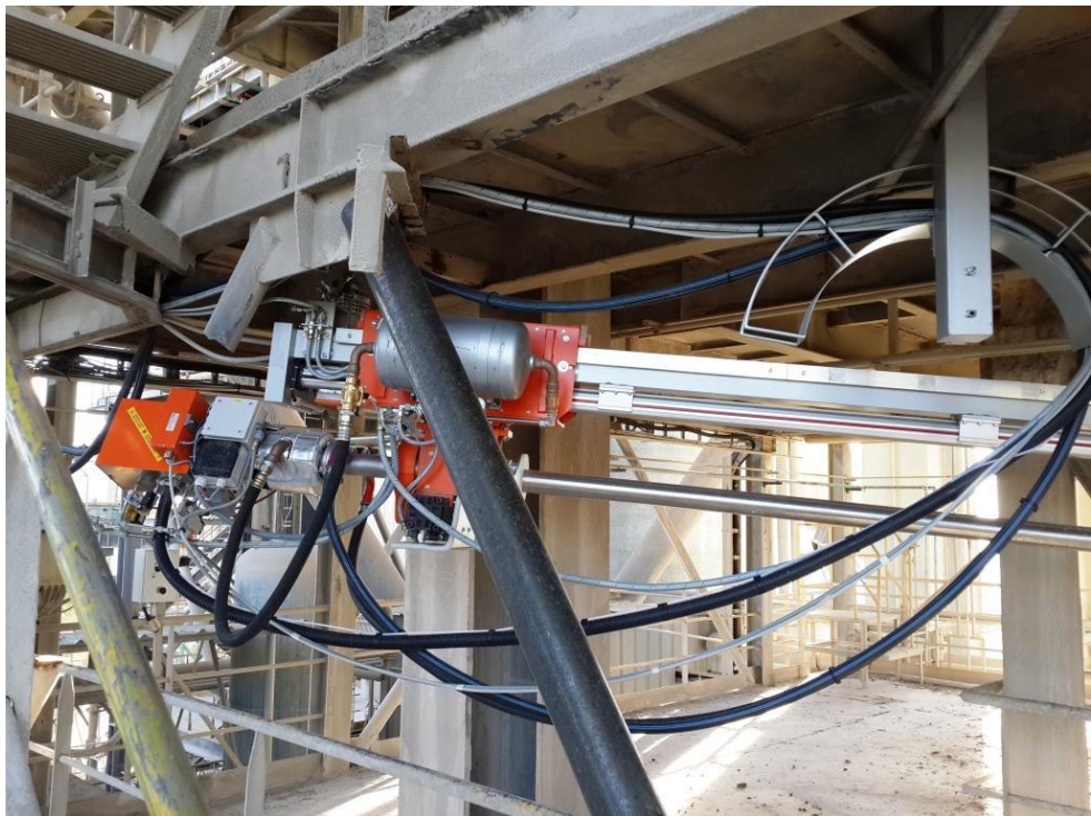
Fig. 37: Probe with cable and hose device completely installed (example)
