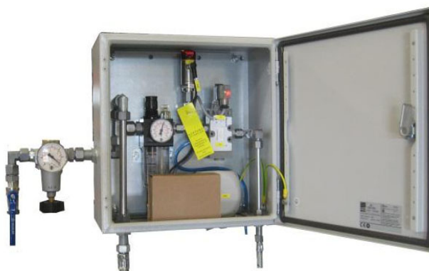
Fig. 14: Pneumatic/compressed air service unit
