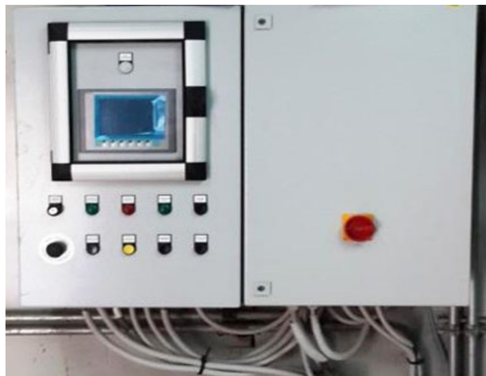
Fig. 36: Installed control cabinet
