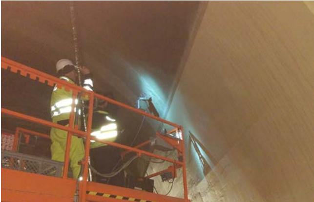
Image 3: Installation of the FLSE200-H sender/receiver unit in the area of the fire location.
