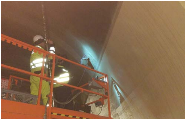
Image 3: Installation of the FLSE200-H sender/receiver unit in the area of the fire location.
