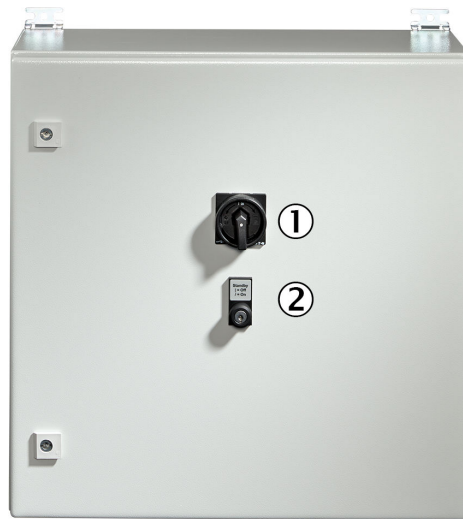
Figure 10: Switches at distributor unit
