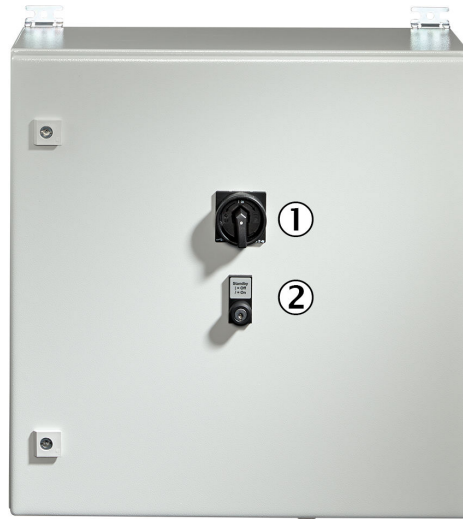
Figure 36: Switches at distributor unit
