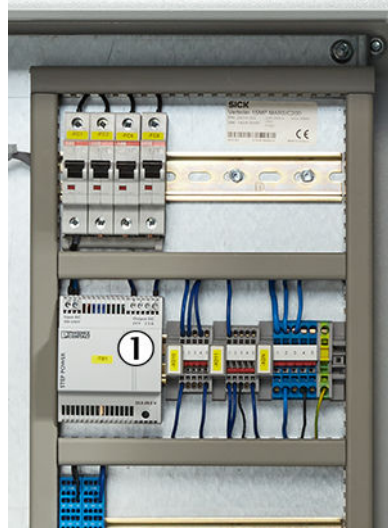
Figure 28: Power supply unit of the distribution unit
