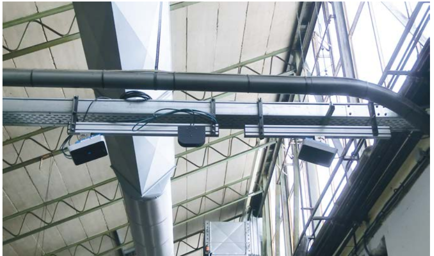
The RFU63x RFID read/write device is installed alongside an external RFA63x antenna above the transport route of the material trolley. It records this information on its way from the warehouse to the pre-completion zones and back.
