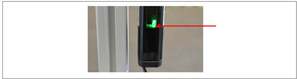
Fig. 119: Checking voltage supply to the light grids
