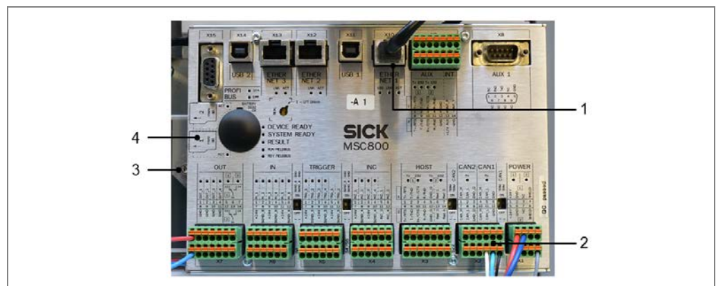
Fig. 139: Unplugging the cables and terminal blocks from the controller
