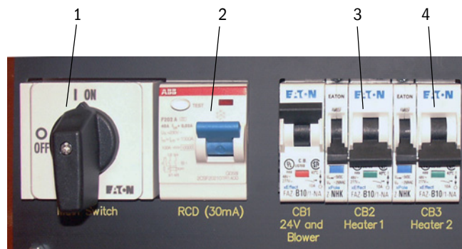
Fig. 66: Main switch and fuses in the control unit
