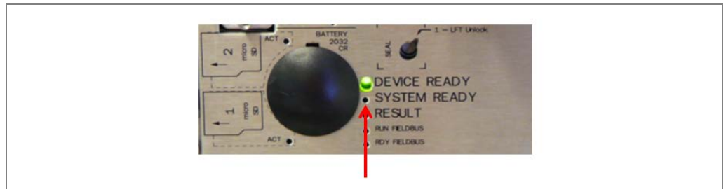
Fig. 105: Fault situation: “SYSTEM READY” LED does not light up
