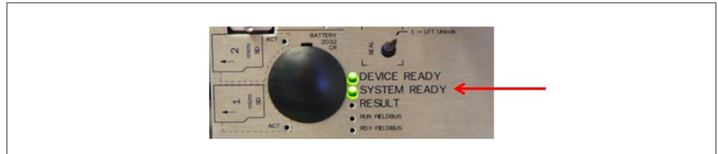
Fig. 103: Fault situation: VMD Ethernet connection
