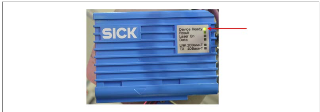
Fig. 79: Checking the operational readiness of the VMD
