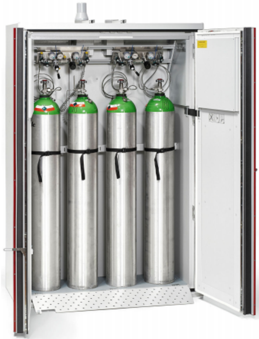
Fig. 28: Gas cylinder cabinet (example)
